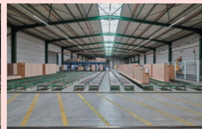
And after the renovation - with new TRILUX light systems.
